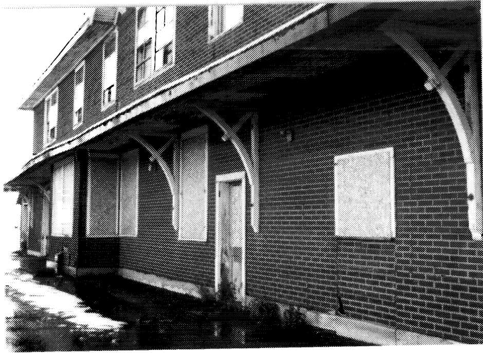
7 NTR Hearst station, use of bracket struts on track elevation. (A. M. de Fort-Menares, 1991.)
