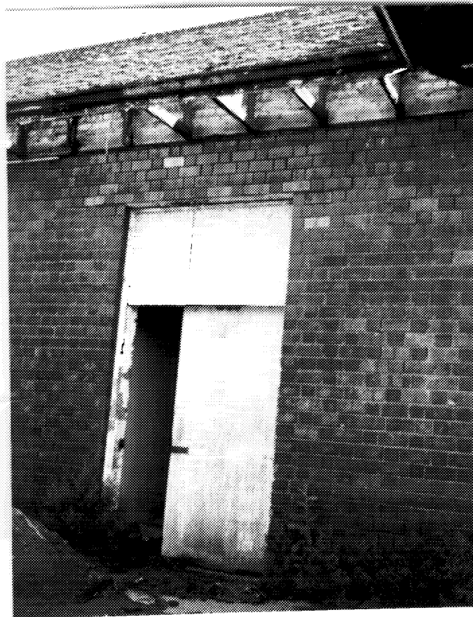
12 CNR West Toronto station, detail of deterioration at the eaves. ( HRSD files, 1992. )
