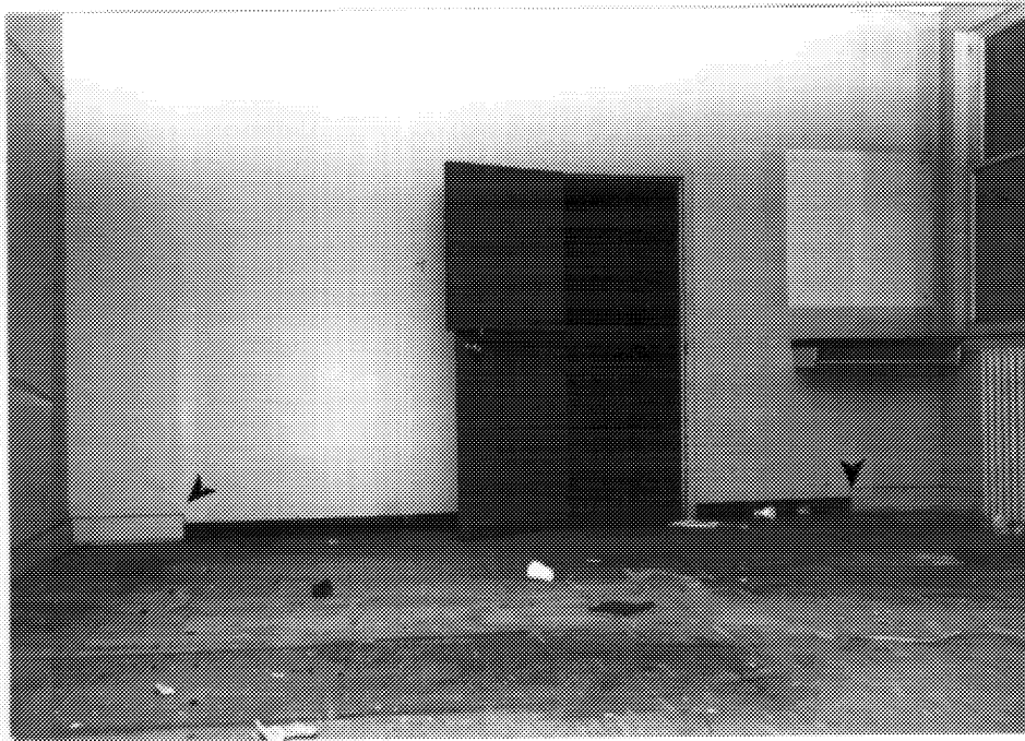
11 CNR West Toronto station, interior of central space looking to a partition wall on the south end that replaced an earlier partition. Early baseboards are visible on each side. ( HRSD files, 1992. )
