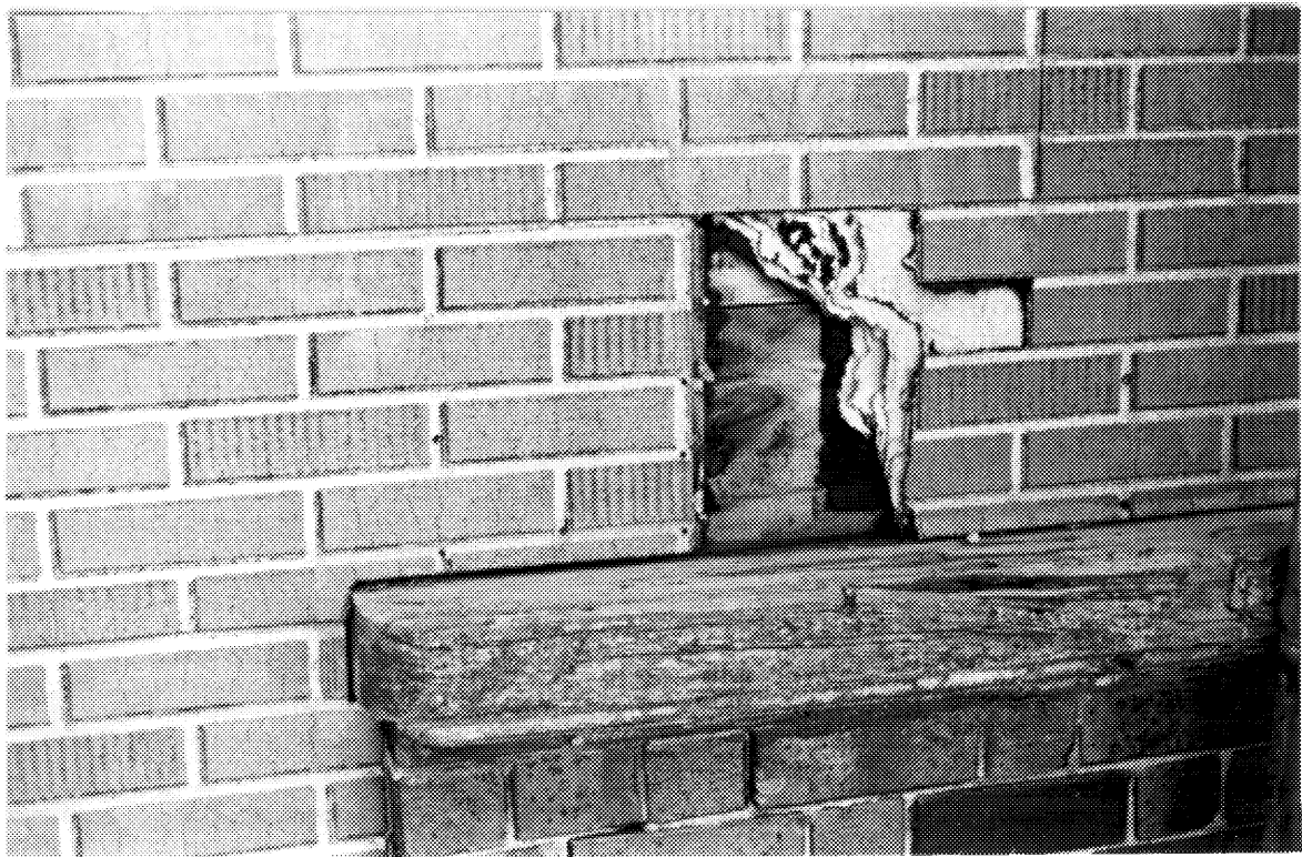
21 Battens were removed from the original siding before it was covered with insulbrick in the 1960s. ( M. Carter, 1993. )
