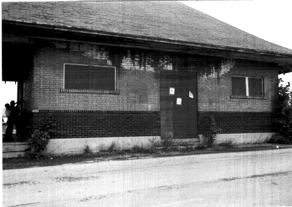
10 Efflorescence on the brick, south side of express building. ( A. M. de Fort-Menares, 1993. )
