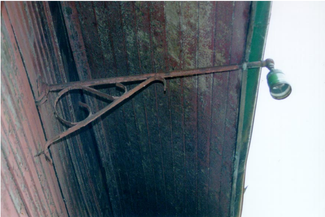
7 Former CNR station, Hespeler [Cambridge], metal light support, track-side elevation. (Murray Peterson, 1997.)
