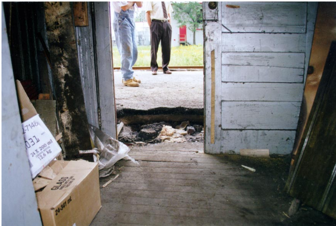
8 Former CNR station, Hespeler [Cambridge], looking north through main door showing the difference between platform and floor levels. (Murray Peterson, 1997.)
